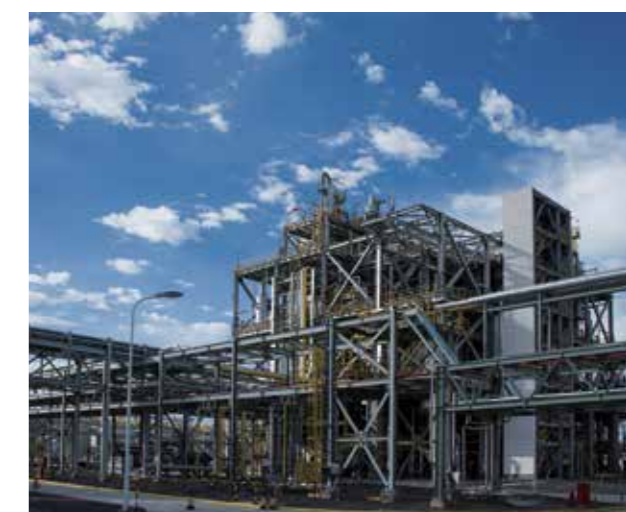
The new PolyTHF facility at Korla site
