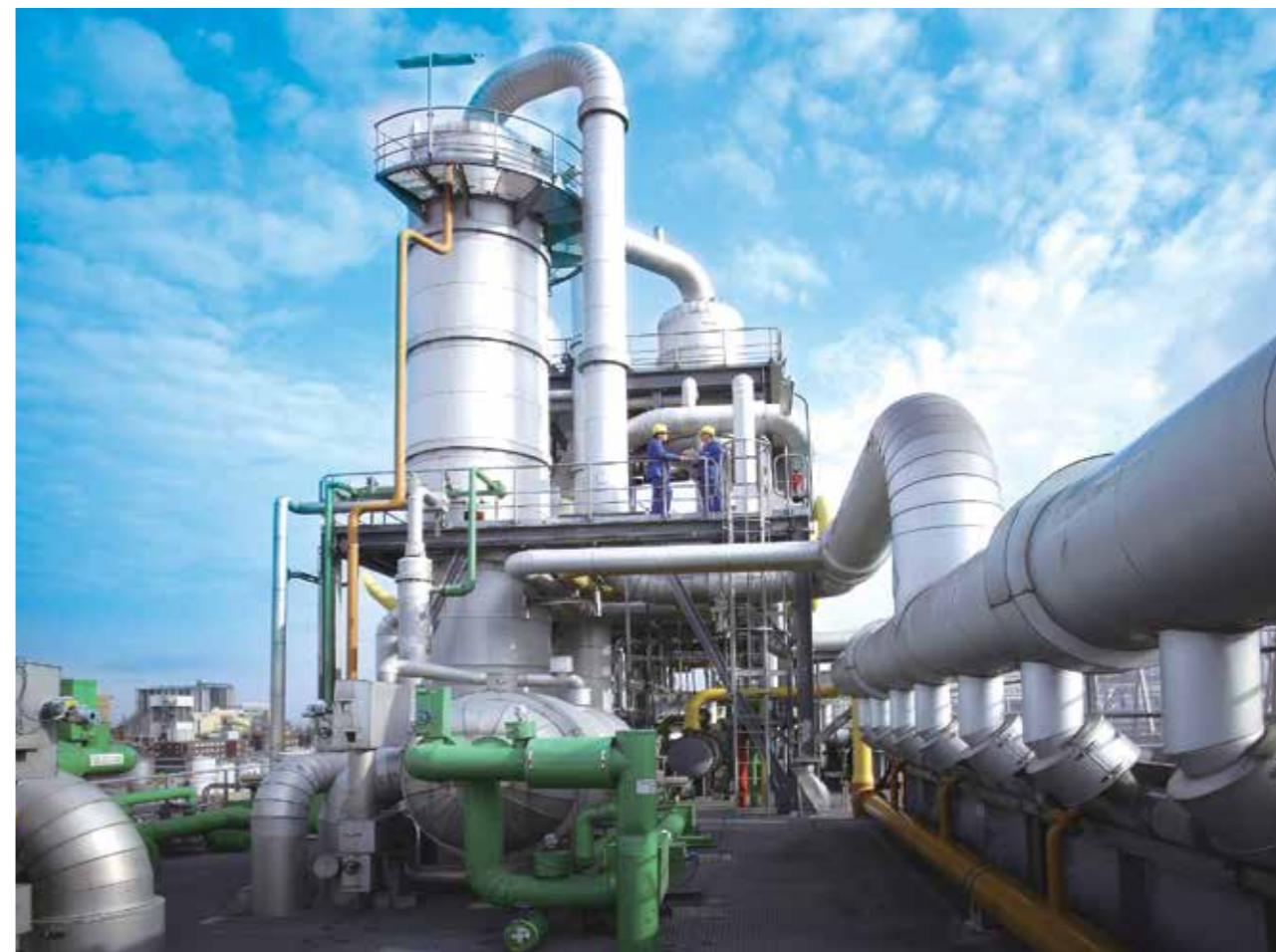
The PolyTHF plant at BASF's Caojing site in Shanghai uses an optimization tool to raise efficiency and save costs.
